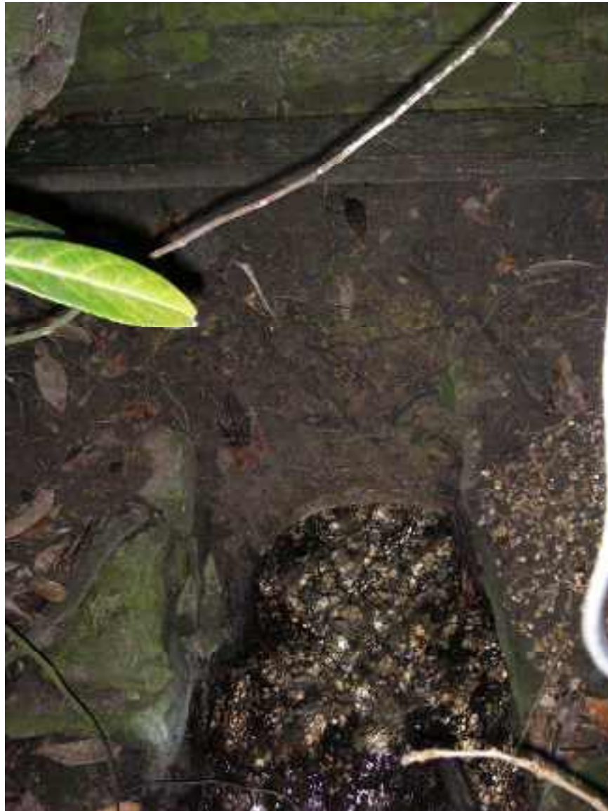
Photo 5 – 450mm diameter pipe discharging to pond
